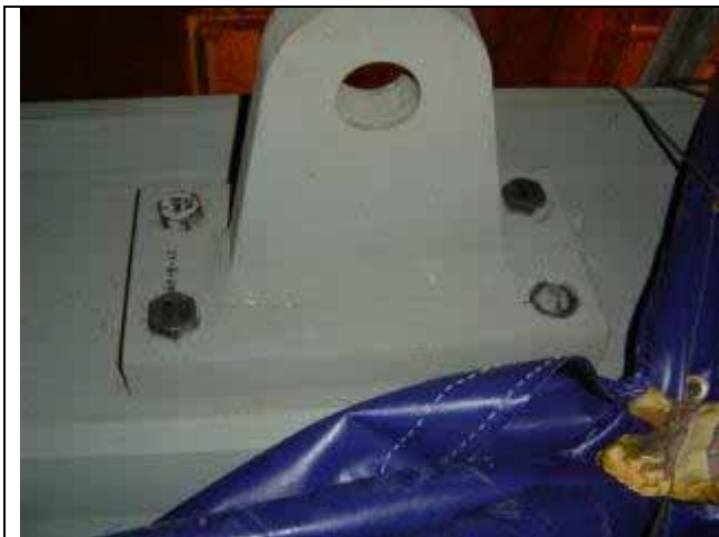
Bolts dislodged on HRSG's Lifting eyelugs
