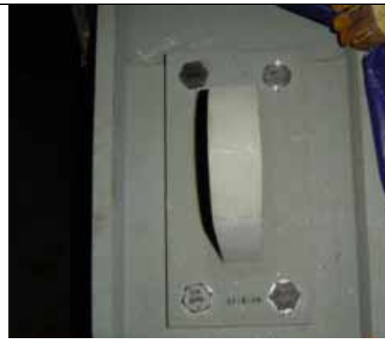
Bolts dislodged on HRSG's Lifting eyelugs
